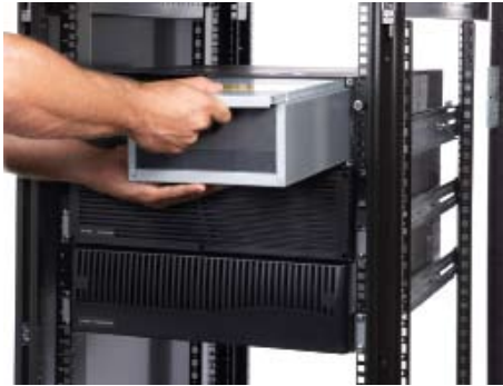
Hot swappable batteries
